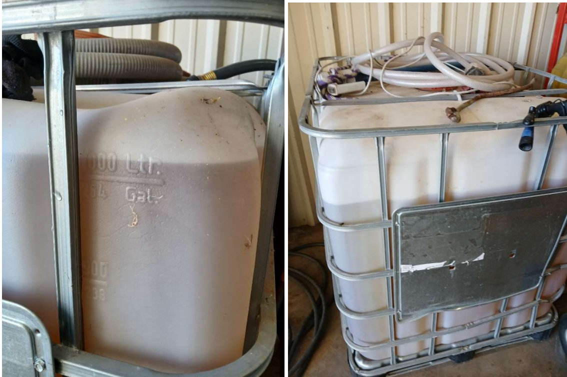
677 Gallons of Fire-fighting foam.
